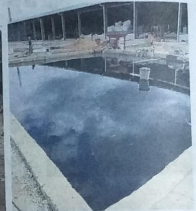
A retention pond to contain wastewater at the factory.
